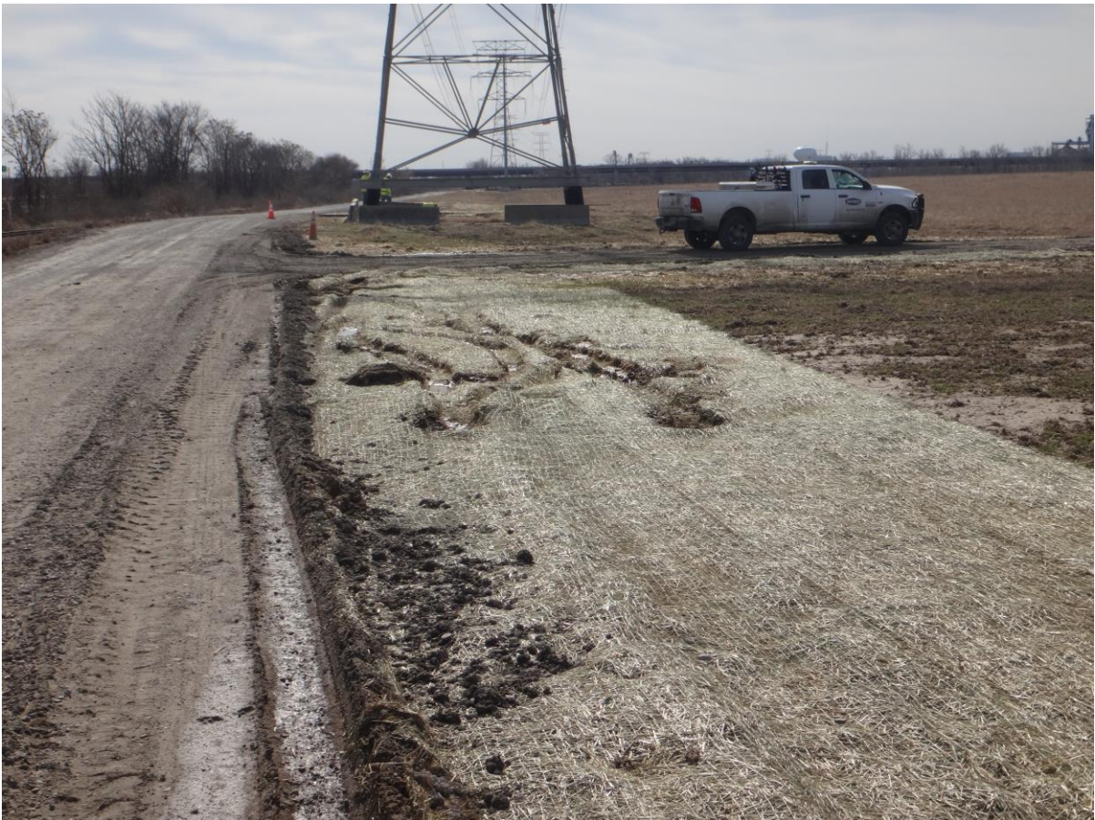
The spring construction for the removal and monopole installation has disturbed a few areas that were stabilized. These areas were currently being repaired with erosion control blanket and seeded.
