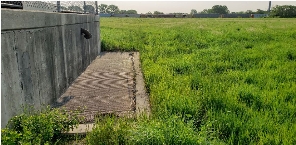
Grating of South Pump Station
