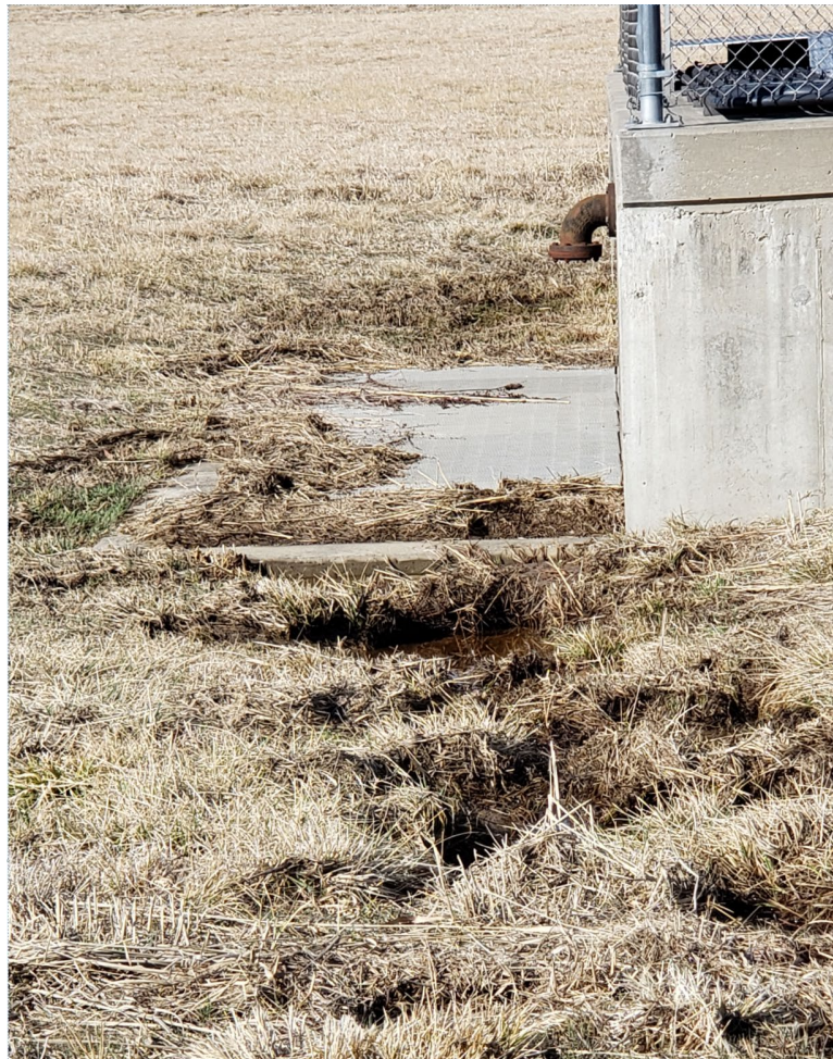
Moderate amount of debris on both the North and South pump station gratings; Minor ground erosion around both stations.
