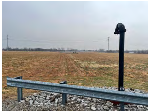
South Pump station, facing east
