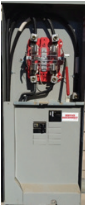
200amp with lever bypass & main disconnect
