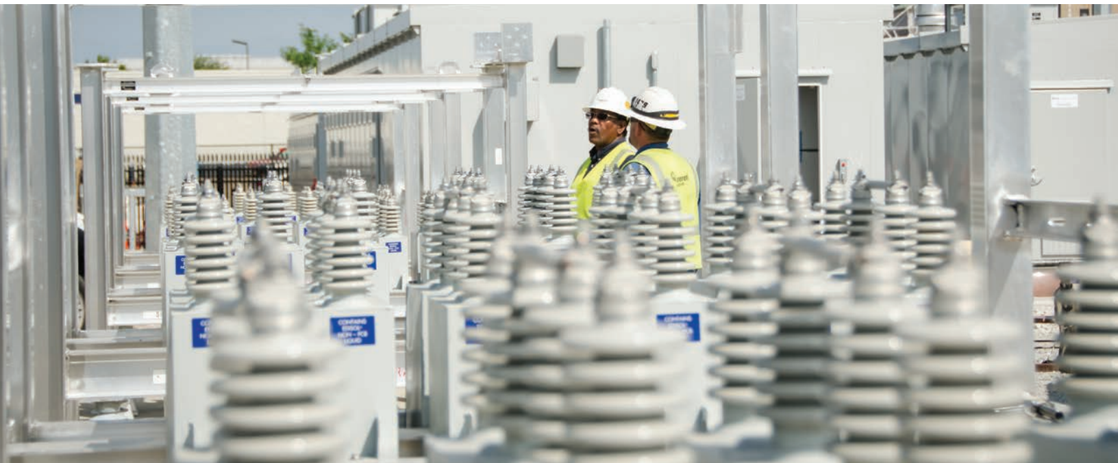
Martin Luther King substation.
